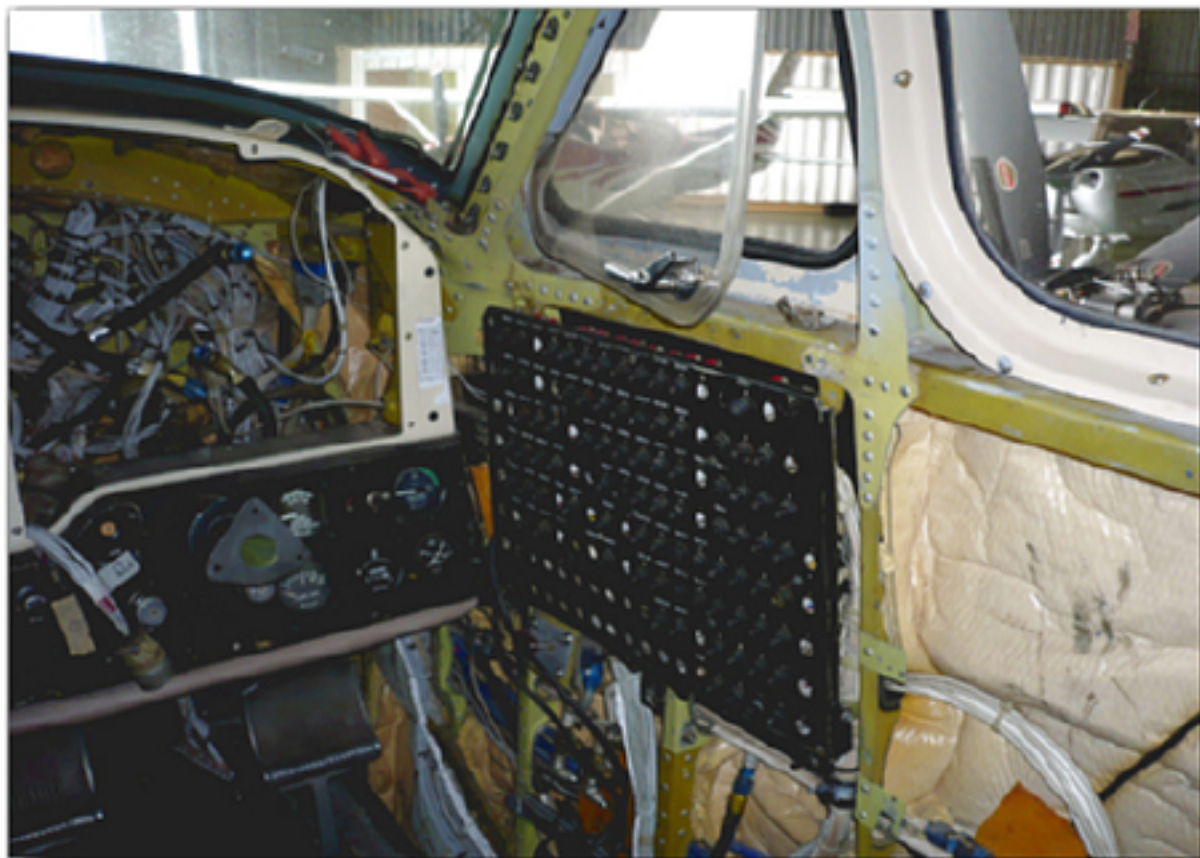
Original circuit breaker panel
